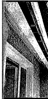
Closed eaves, vents not screened with 3-millimetre mesh (1 pt)
